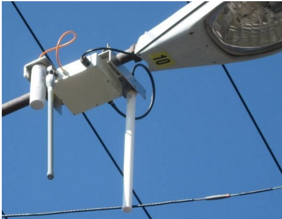
Figure 5.2: CitySense node deployed on a street lamp. The thick antenna pointing downwards on the right side is connected to the 900MHz backhaul radio, and the thinner antenna on the left side is connected to the 802.11 sniffer radio. The node is powered from the streetlight.
